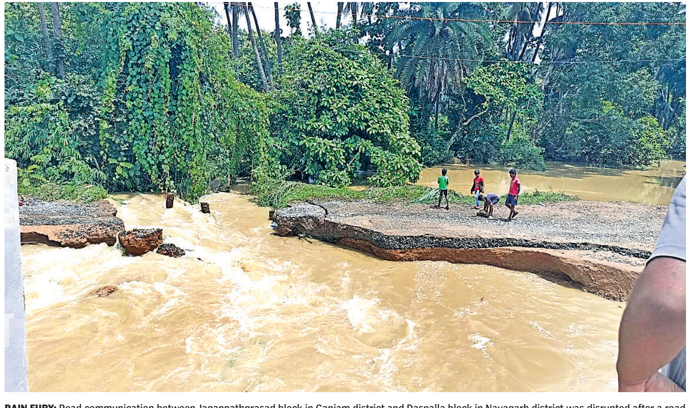
RAIN FURY: Road communication between Jagannathprasad block in Ganjam district and Daspalla block in Nayagarh district was disrupted after a road passing through Kadua panchayat was washed away following torrential rainfall in the wee hours of Sunday
